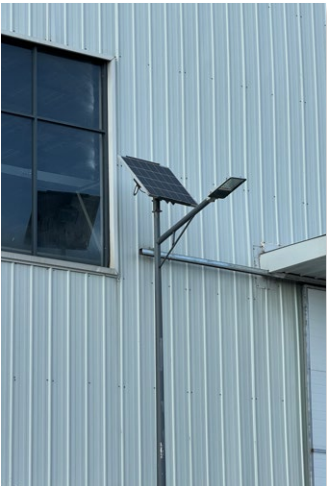
Intelligent PV lighting
